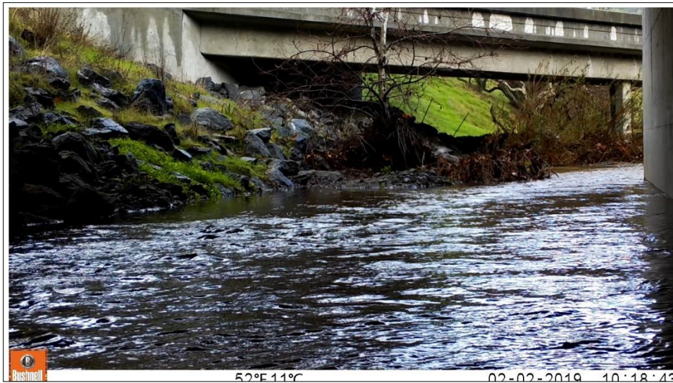
Figure 16. Cedar Creek bridge flooded during February 2019.
