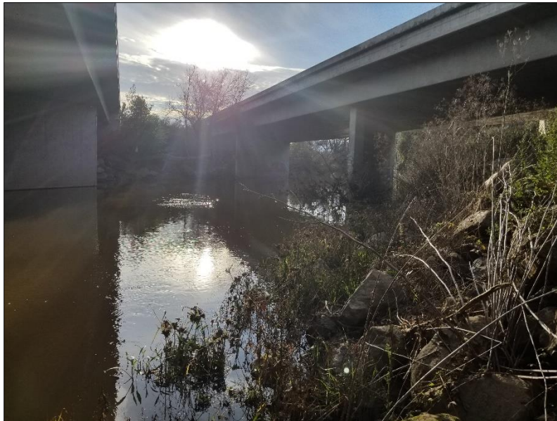
Figure 15. Pacheco Creek bridge flooded during February 2019.
