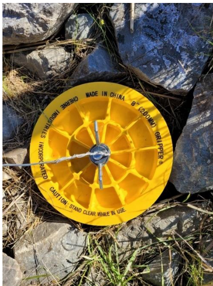
Photo 33. Removeable caps, added to the quick drain pipes to prevent leakage (photo provided by SCVHA, November 30, 2021)
