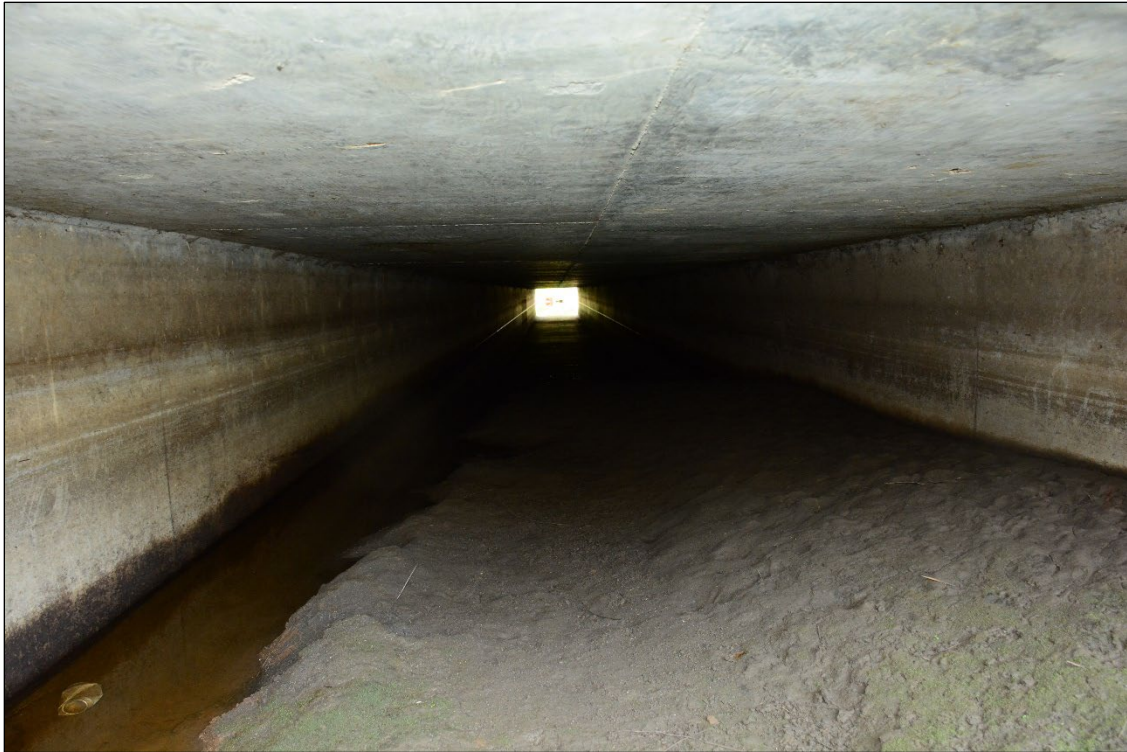
Figure 8. Coyote Alamitos Canal at Santa Teresa Boulevard, mid-section on 1/13/2021.
