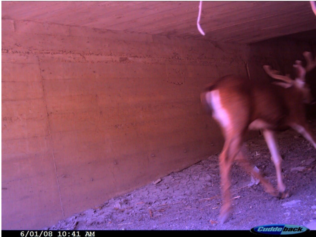
Figure 14: Deer crossing beneath the Bailey Bridge at Fisher Creek on 6/1/2008, from the south most eastern section of the bridge.
