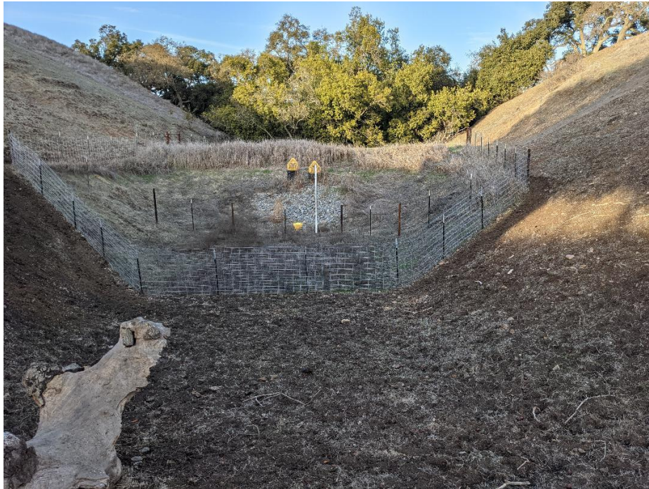
Photo 37. Completely Dry Pond Bed at CR1 (December 29, 2020)
