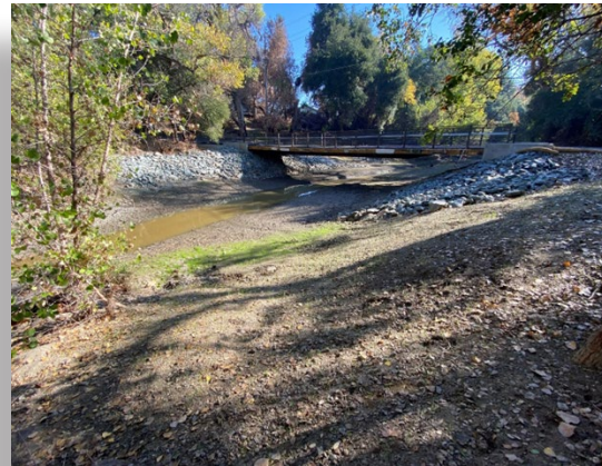
Coyote Creek at Singleton Road Crossing prior to bridge installation (left) and after installation (right), looking upstream.
