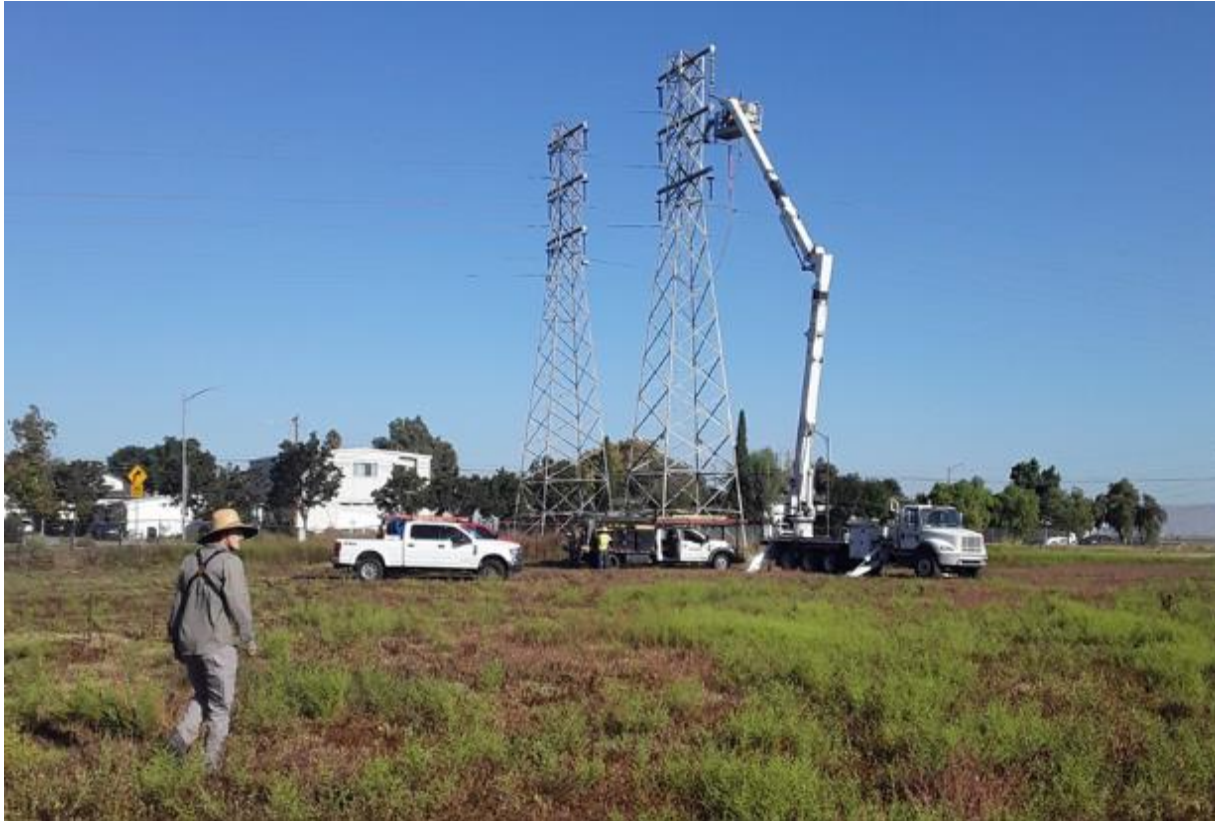
Figure 13. In October 2023, subcontractors for PG&E entered the Cisco site and conducted maintenance work on an electrical pylon on the north-end of the site.
