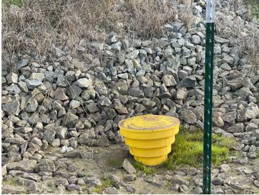
Photo 32. No water at CR4 due to open drain valve (photo provided by SCVHA, February 10, 2021)
