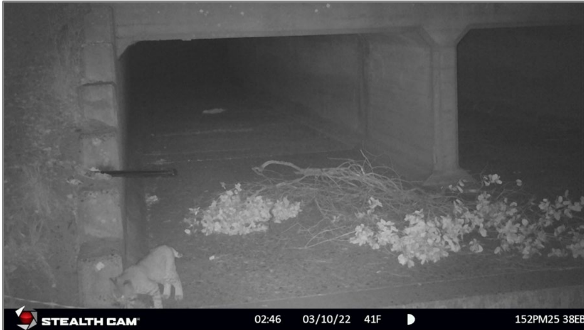
Figure 32. Bobcat successfully crossing through C10 Killdeer Creek bridge (370060)/Elephant Head Creek Culvert
