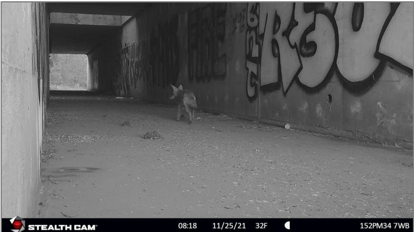
Figure 87. A coyote crossing through SR-152 culvert C22 PM 34.7.
