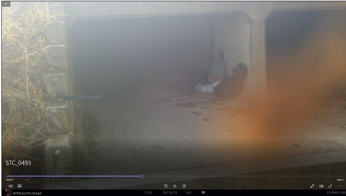
Figure 34. Trespasser at the C10 Killdeer Creek bridge (370060)/Elephant Head Culvert
