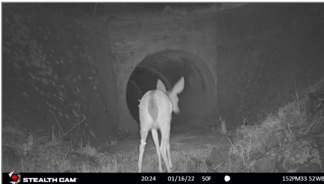
Figure 82. Deer approaching SR-152 culvert C21 PM 33.52 on January 16, 2022.
