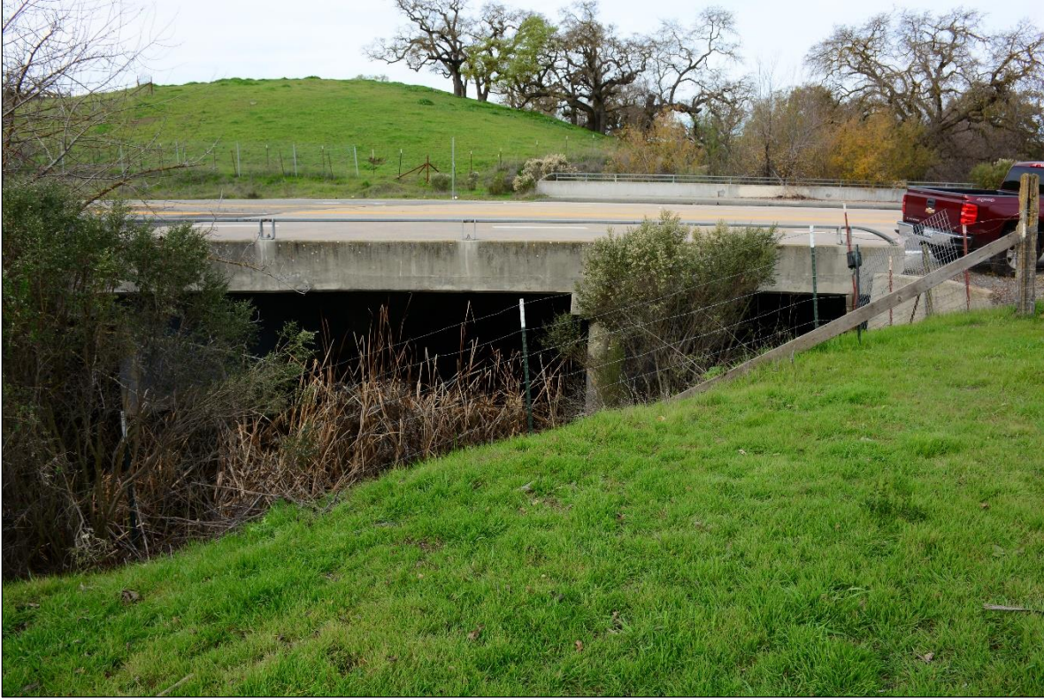
Figure 115. Bailey Bridge at Fisher Creek on 1/14/2022, south side of the bridge, eastern section.
