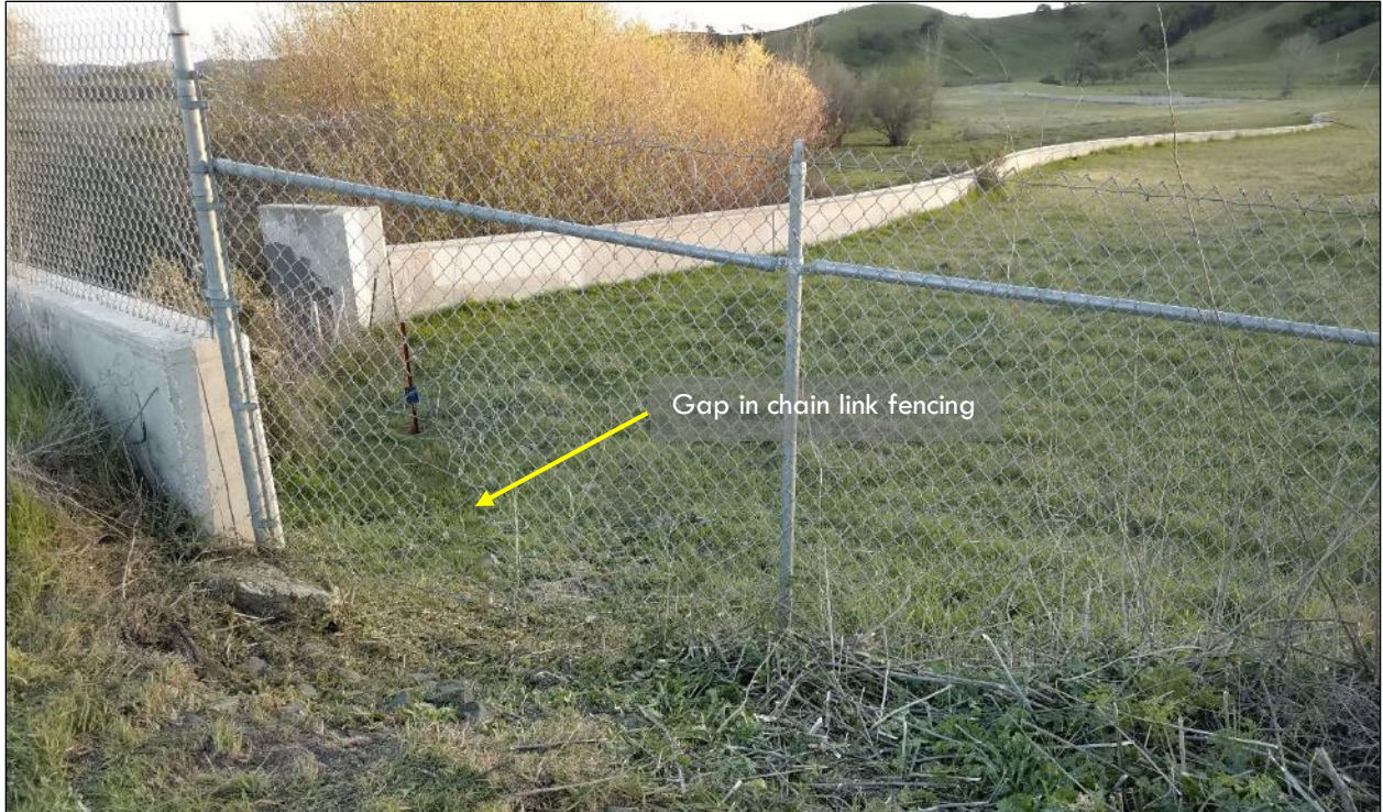
Figure 10. Gap in chain link fence near Fisher Creek Culvert.
