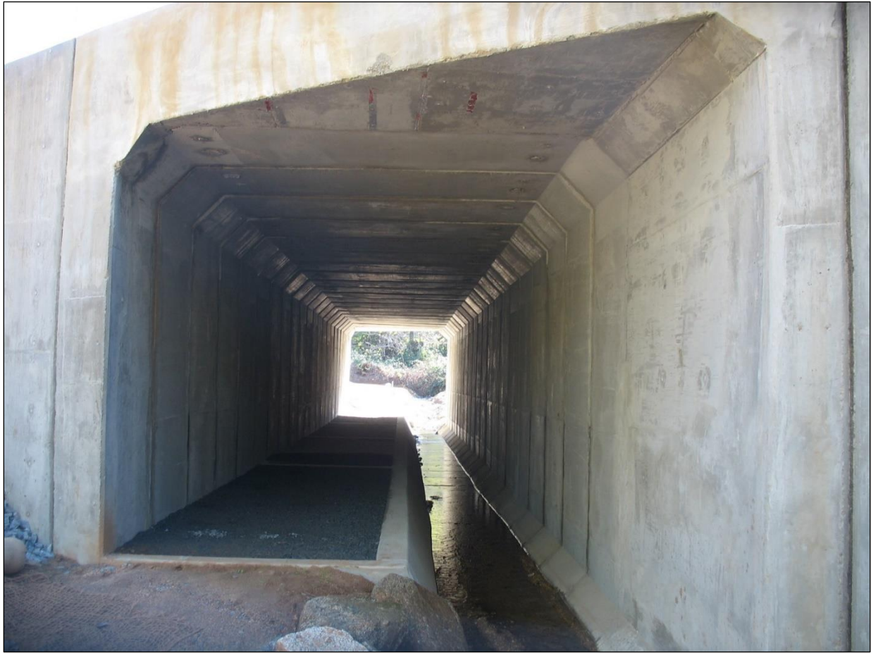
Figure 116. Culvert retrofit on SR-89 by Ken Russo, Senior Environmental Planner, Branch Chief Unit M5, Resource Biologist, Caltrans, District 3.
