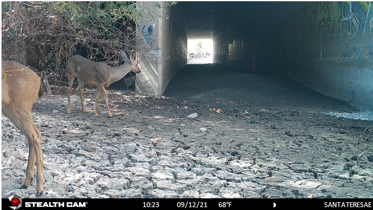
Figure 76. Deer on the west side of the Santa Teresa Blvd. Fisher Creek dual box culvert.
