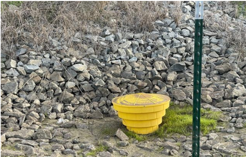
Photo 69. No water at CR4 due to open drain valve (photo provided by SCVHA, February 10, 2021)
