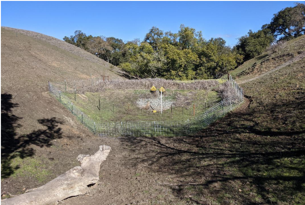
Photo 56. Completely Dry Pond Bed at CR1 (February 1, 2021)
