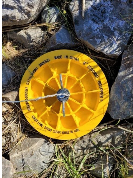
Photo 70. Removable caps, added to the quick drain pipes to prevent leakage (photo provided by SCVHA, November 30, 2021)
