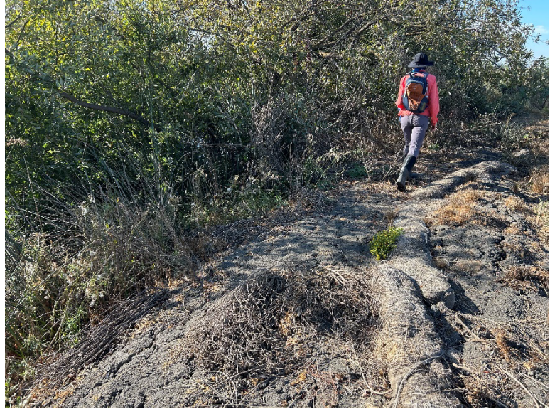
Photograph 1. Potentially unstable right bank segment in Reach 2a (Erosion Feature #6).
