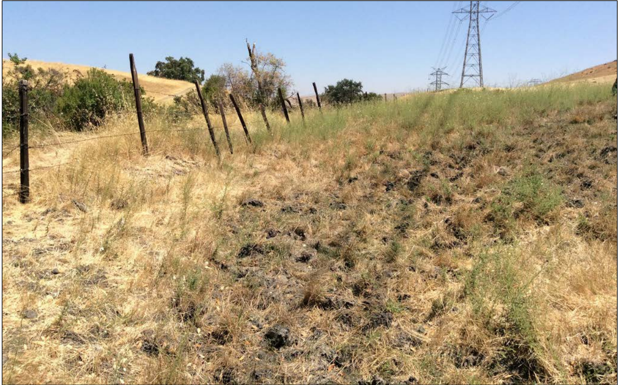
Photo 29. Year 1 Conditions at Photo Point 12 during Vegetation Monitoring, Where the Hillside Seep Collection Ditch was Enhanced in the Seep Collection Area (August 8, 2017)
