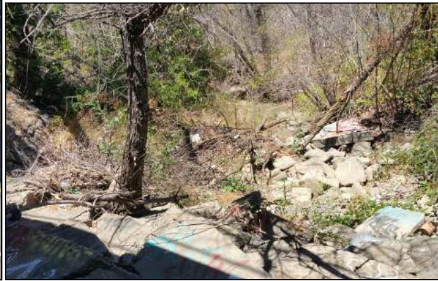
Figure 21: Debris at Monterey Road Culvert.
